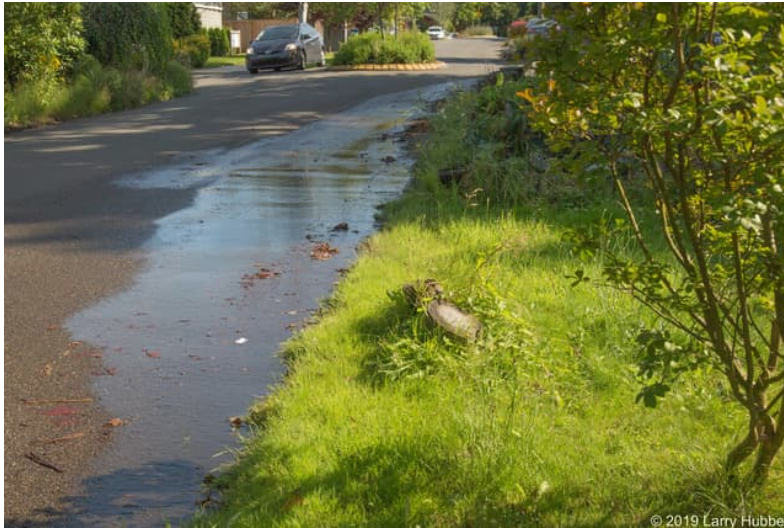
Figure 6 – Seep at 28th Ave East (between E. Aloha and E Ward Streets)
